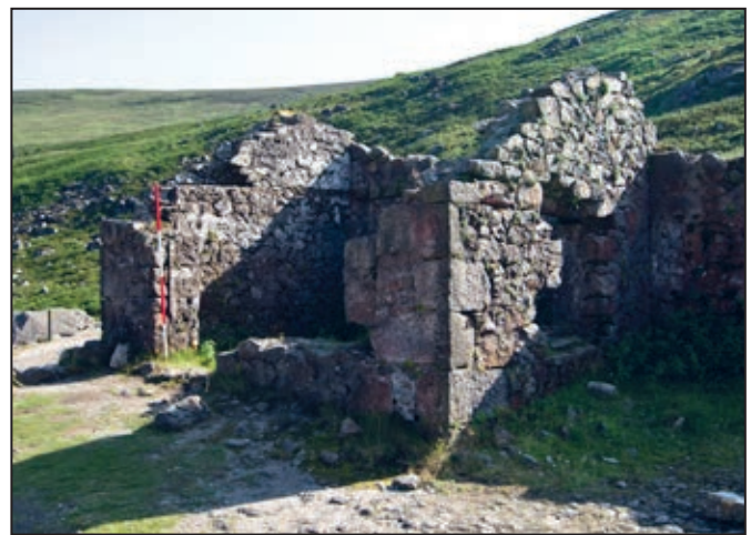
Figure 19. This office was built in the 'mine yard' after the Old Hero dressing floors were revived in the late 1860s
