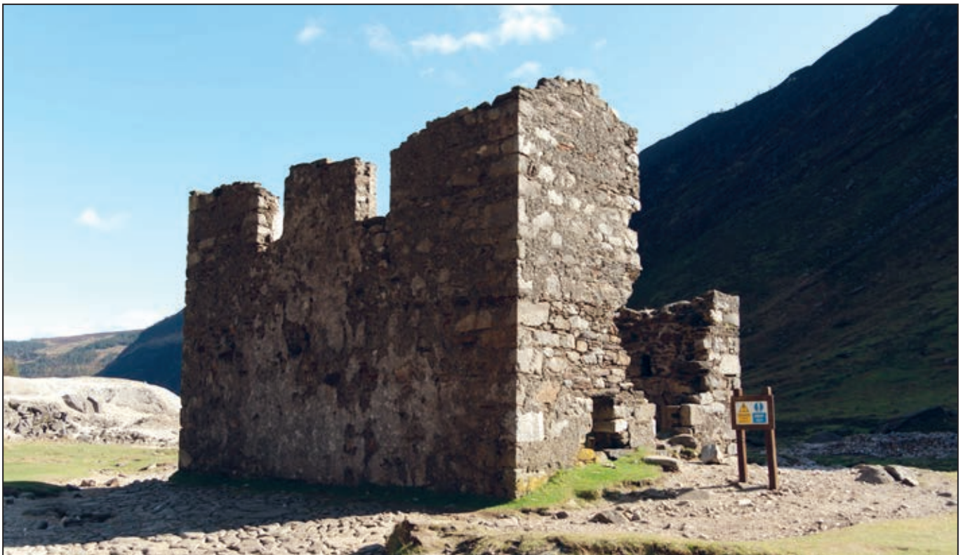
Figure 28. The Cornish rolls crusher house still dominates the site today as it did 150 years ago. Its conservation is a matter of urgency
