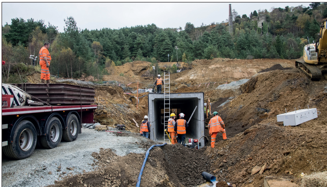
Fig. 18: Emergency works being undertaken without planning permission by Irish Rail at White Bridge, Tigroney, in October 2014. Sub-surface archaeology was exposed and damaged by heavy earth moving machinery and large quantities of mine spoil were moved around the site, disturbing rare mineral exposures. Wicklow County Council was forced to issue an enforcement notice on Irish Rail to stop the works. Image, Martin Critchley, 2014
