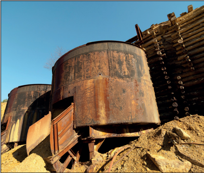
Fig. 19: The iconic ore bins at Tigroney dating to the 1960s which, after pressure was brought to bear on the DCENR, will now be properly conserved. The surrounding spoil is however, earmarked for removal, thus degrading the authenticity of the site. Image, Martin Critchley, 2012
