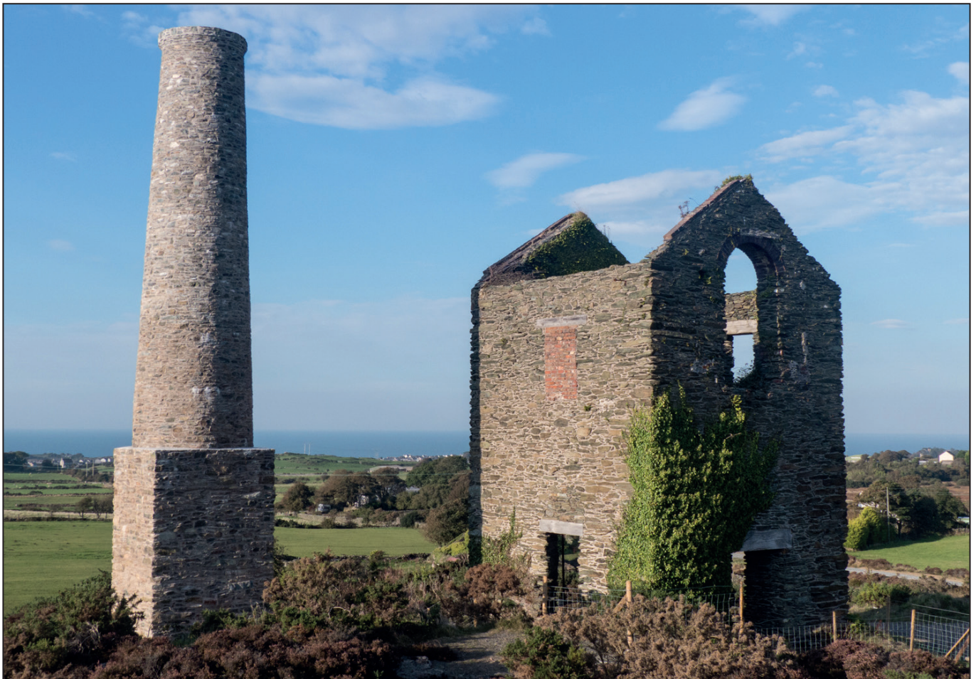
Fig. 8: The Pearl Engine House, the earliest surviving Cornish-type engine house at a Welsh metal mine, is an iconic feature of the historic mining landscape of Parys Mountain, and a vital part of the UNESCO GeoMôn Geopark. The chimney (left) collapsed in 1982, and was rebuilt in 2012-13. Since this photograph was taken, the engine house (right) has been consolidated and re-roofed, and will serve as a small interpretation centre.
